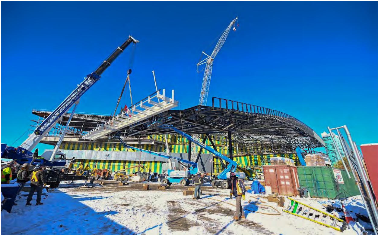
Leading edge of the canopy at the BMO Centre Expansion rising in Calgary, image courtesy of CMLC and Calgary Stampede
