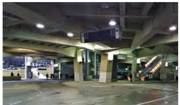
Fig. 1: Transfer girders at the Paul S. Sarbanes Transit Center in Spring City, MD, USA (photo courtesy of Evan Bentz)
