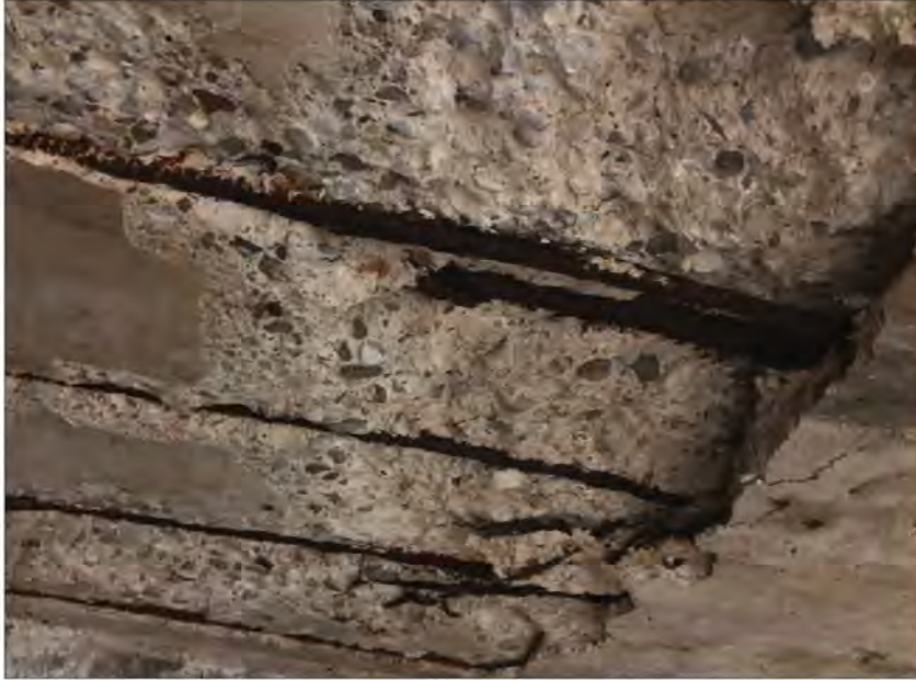
Structural deterioration as a result of a failure of the podium deck waterproofing system.
