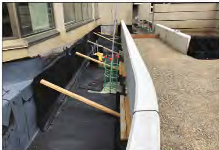
Cross-sectional view of overburden installed on a podium deck at a condominium located at 30 Greenfield Avenue in Toronto.
