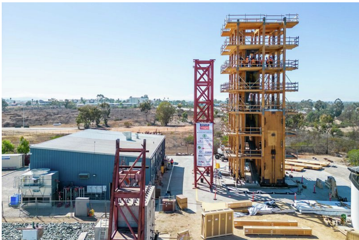
Crews prep for the Natural Hazards Engineering Research Infrastructure (NHERI) TallWood research project in San Diego. – LEVER Architecture
