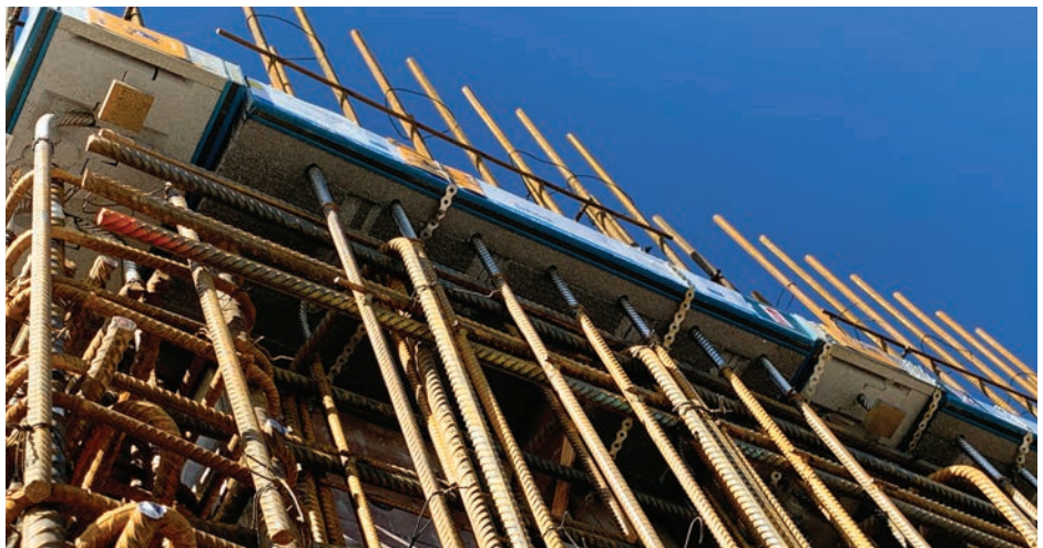
The fire hall tower has a sturdy reinforced concrete frame to resist seismic loads. Isokorb® structural thermal breaks maintain structural integrity while reducing heat loss at the penetration by up to 90 percent.
