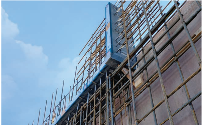
Vertically and horizontally oriented thermal breaks at the parapet atop the tower prevent warm interior structures from dissipating heat energy into the environment.
