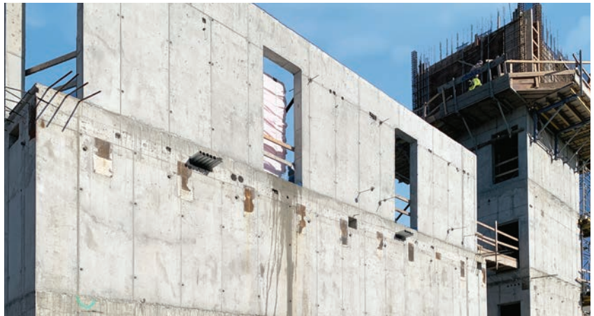
The main building at left and the training tower at right are structurally integrated on four levels but thermally isolated with Isokorb® concrete-to-concrete and concrete-to-steel structural thermal breaks.
