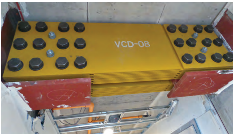
Top: Rigid steel placeholder to be replaced with a VCD unit. Bottom: A VCD unit in place.
