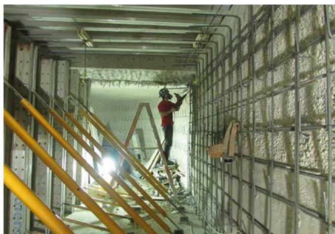
Ensuring the safety of personnel in the enclosed influent channels adds to the complexity of an already challenging project.
