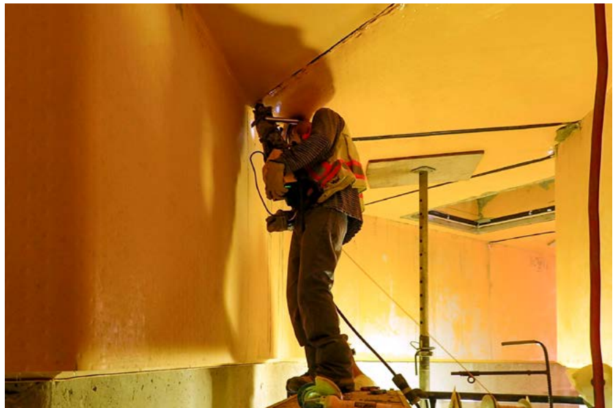
Field welding of the HDPE liner was done with an extruded welding rod of the same HDPE material.
