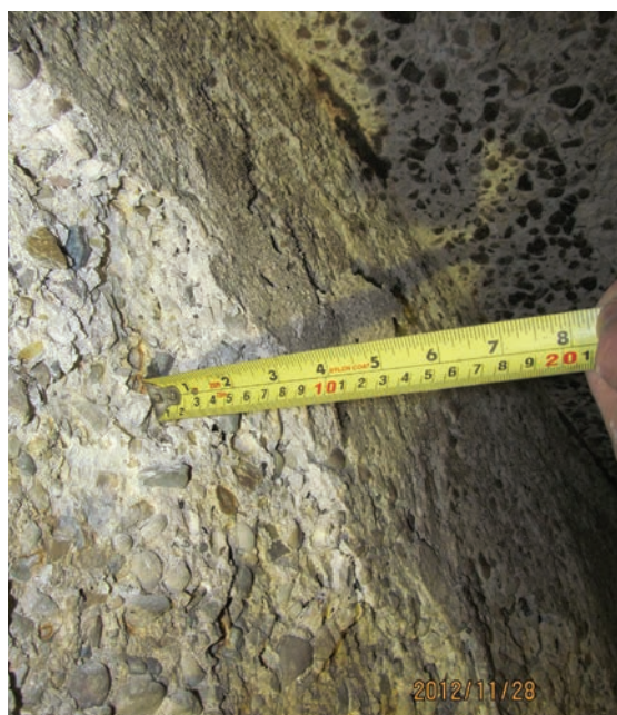
Fig. 1: Extensive depth of concrete deterioration on channel walls
