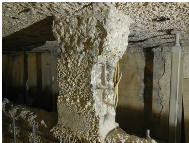
Fig. 2: Existing column deterioration
