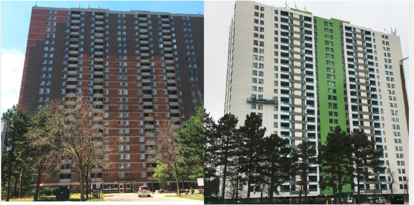
-Teesdale Place: Before (left) and after (right) undergoing a building façade restoration
