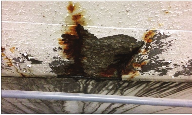
Deterioration as a result of waterproofing failures.
