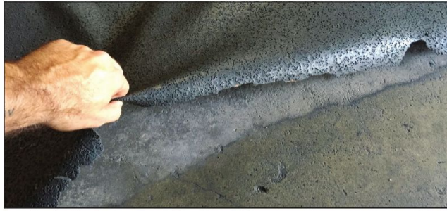
Wearing, debonding, and general system failure of a thin traffic deck coating is shown in the image above.
