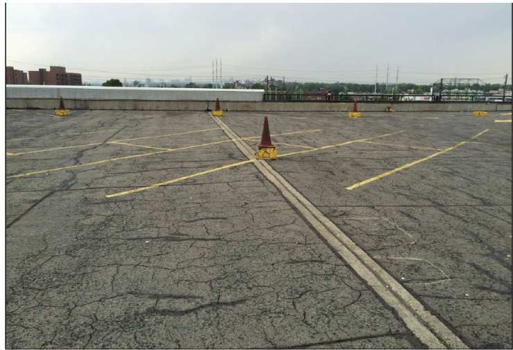
An example of deterioration of a thick waterproofing system on a roof deck.
